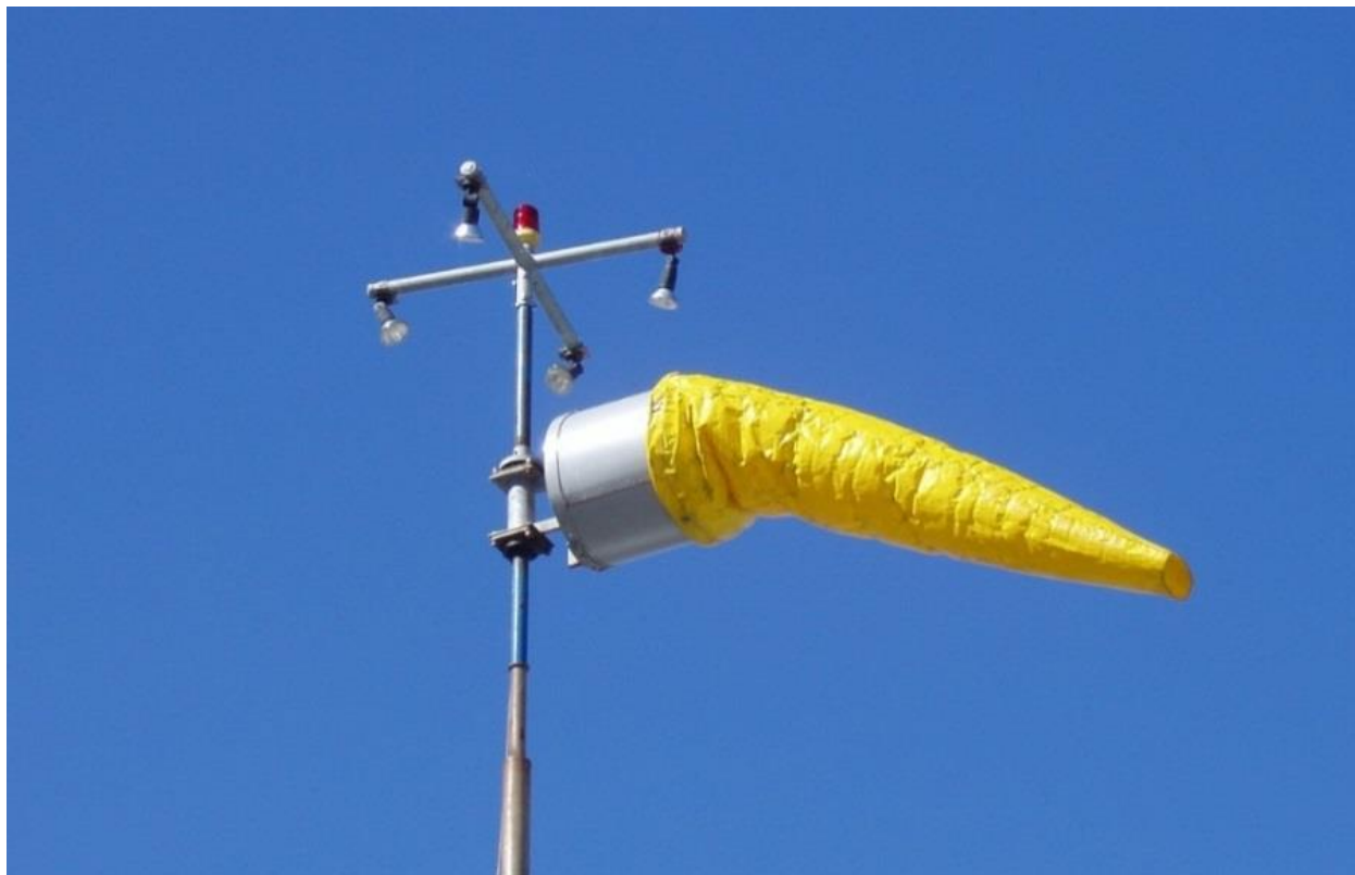
Figure 10: Windssock and Lighting
